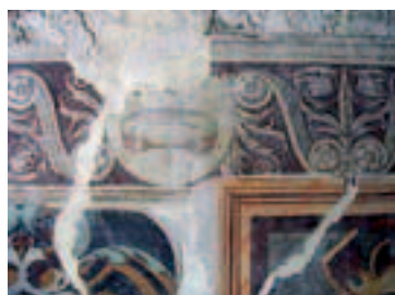
Fig. 7.2 - 7.3: Loggia, first floor; west elevation – detail, blocked apertures and painted plaster sequences.
